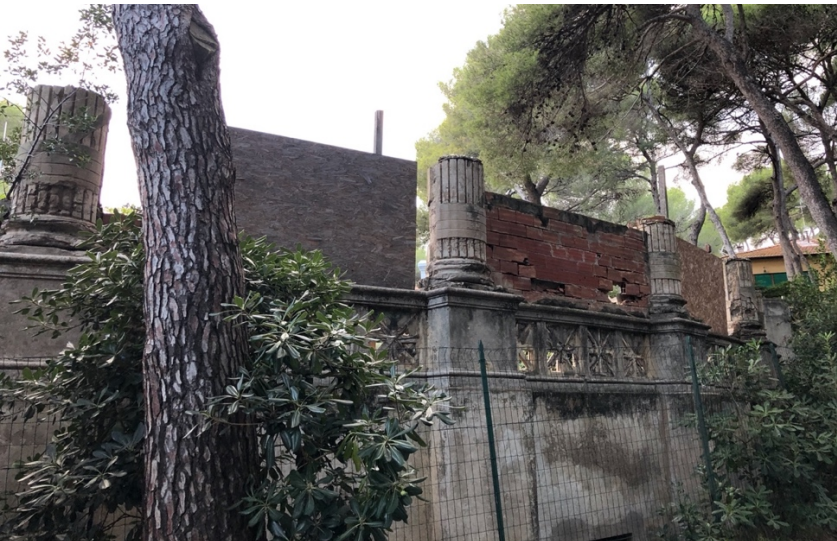
Figure 68 - The arena in the backyard with the severed columns. Source: photo of the author.
